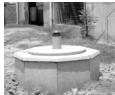
The rainwater harvesting system at ZRC
